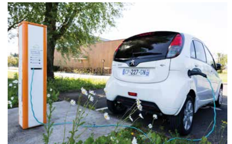
Charging stations for electric vehicles at the South Environmental and Sustainable Development Resource Centre - Paris-Orly
